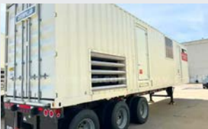
2005 2,000kW CAT Genset Sold for $489,780 in Vestal
