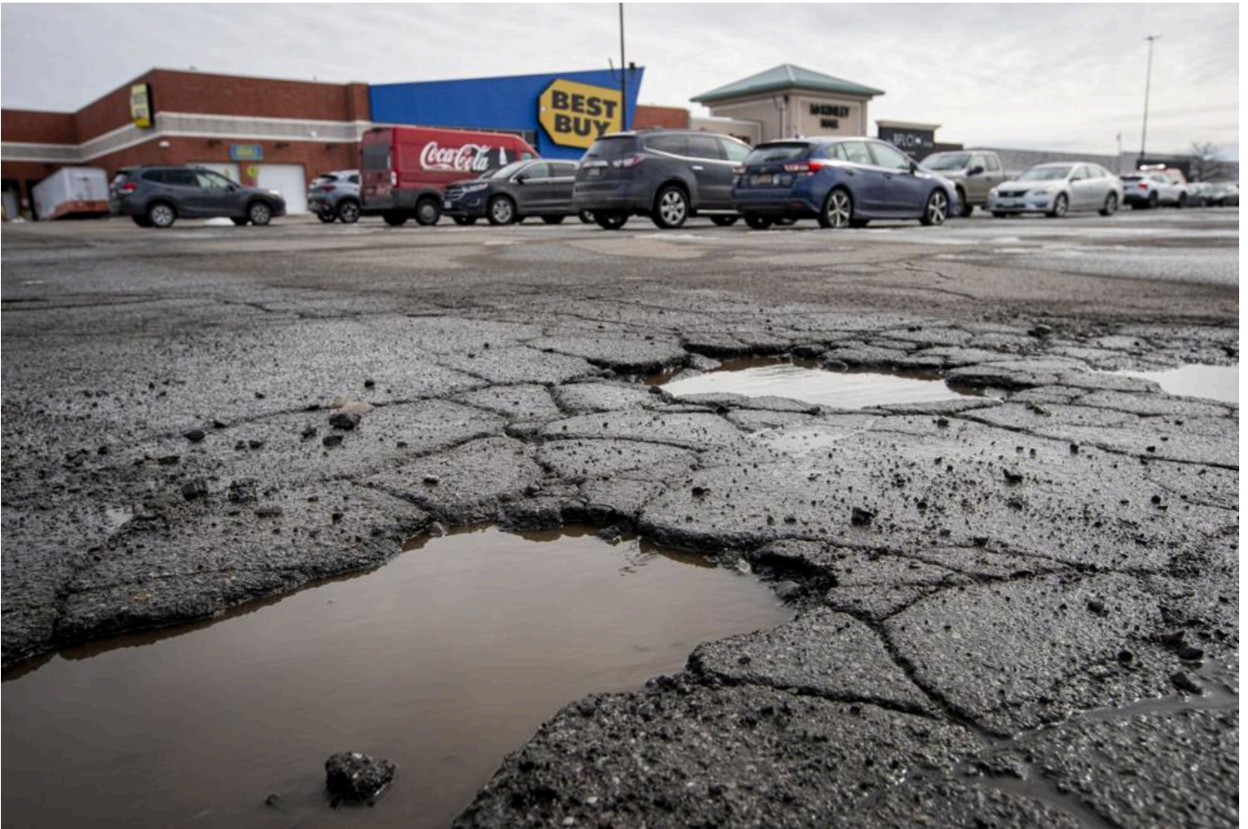
Water fills potholes in the parking lot of the McKinley Mall.
